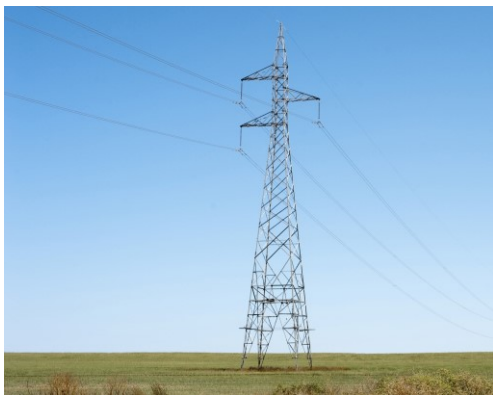
Figure 7. A typical lattice frame electricity transmission tower. (www.freeimages.co.uk)
