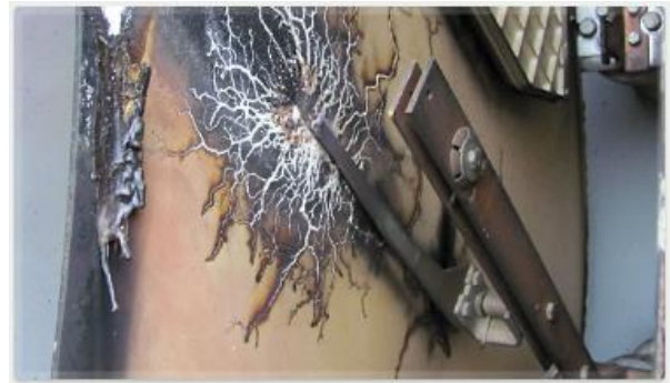
FIGURE 3.4 TRACKING DUE TO DISCHARGE IN SWITCHGEAR [78]
