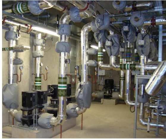
Figure 6: The system circulating pumps installation. Heating and chilled water header circuit pumps are in the foreground and the ground loop pumps in the background.
