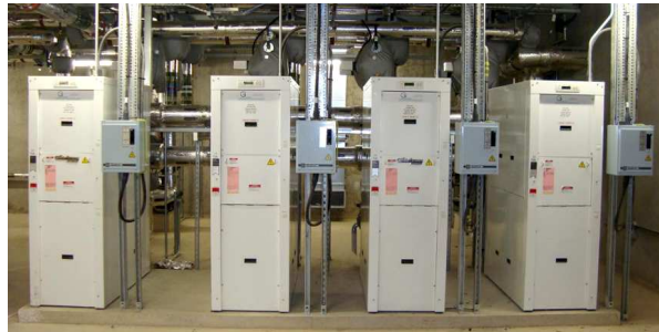
Figure 4: The heat pump installation in the basement plant room.
