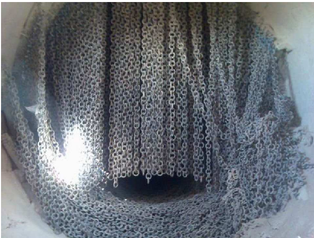
Fig. 2 A real image of chains curtain inside rotary cement kiln at Kufa cement plant . Courtesy of Kufa cement plant (image no. CK-005)
