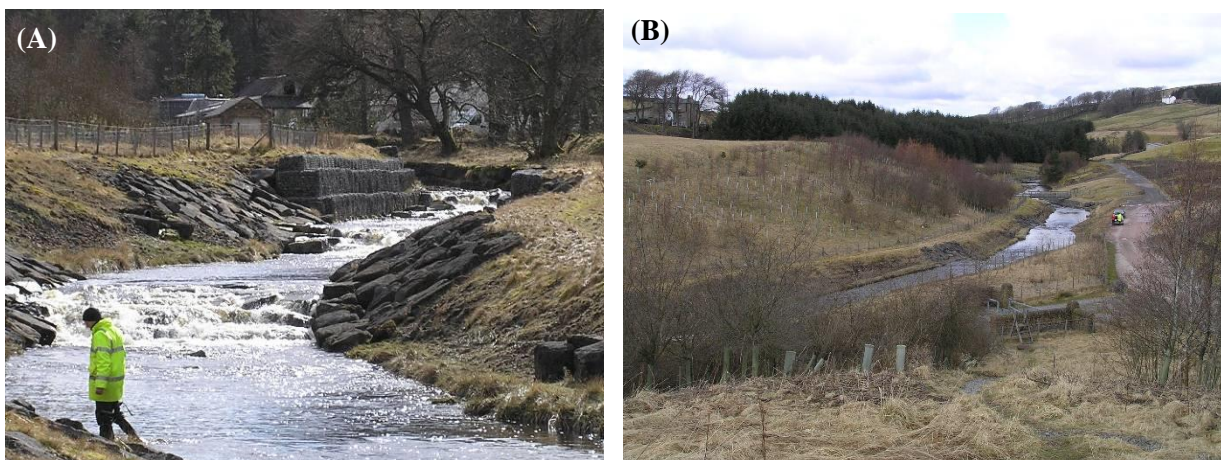
Figure 2. Use of gabions to stabilise banks of the River Nent, Cumbria (A) and re-grading, capping and vegetation of spoil material along the same stretch of river (B)
