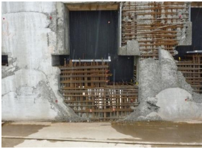
Figure 1.2: Pitfalls of conventional concrete with dense reinforcements [7]
