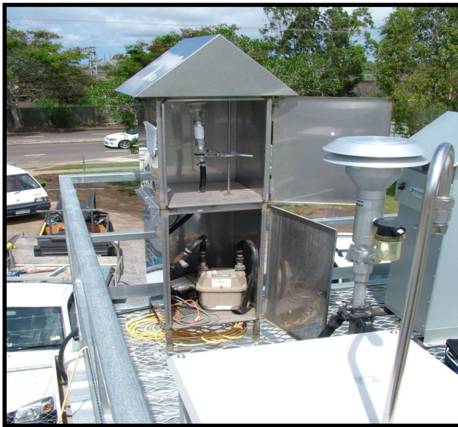
FIGURE 2 A LOW VOLUME AIR SAMPLING CHAMBER SITED ON THE ROOF OF THE SOUTH GLADSTONE AIR MONITORING STATION
