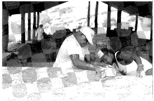
Figure 4 Hobson Levi shows the chairman of neighbouring Boigu Island how to lay mud bricks. [Photographer: P. Haar, 1987.]
