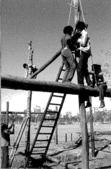
Figure 1 Previous work experience at Top End cattle stations had equipped the Mt Catt mob for the challenge of hoisting heavy pole timbers into the roof structure. [Photographer: P. Haar, 1987.]
