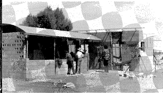
Figure 2 Renovation of a Kingstrand Hut (left) at Yuendumu in Central Australia. These transitional houses were built during the 1960s and are shown here being upgraded and extended during September 1987 to better suit community needs. [Source: AERC, University of Queensland. Photographer: P. Memmott.]
