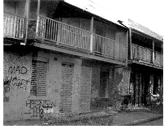
Figure 1 Louis Street in Redfern showing the wear and tear on the Aboriginal Housing Company's terrace houses. [Photographer: P. Vallis.]
