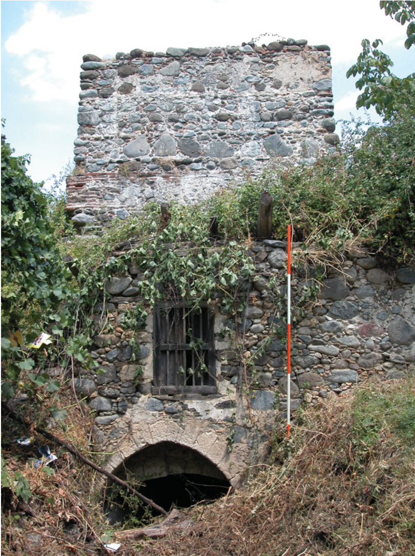
Figure 7 Lachistos mill: penstock (above), milling room (with window) and turbine room (with arch) (Chris Parks). (Colour online)
