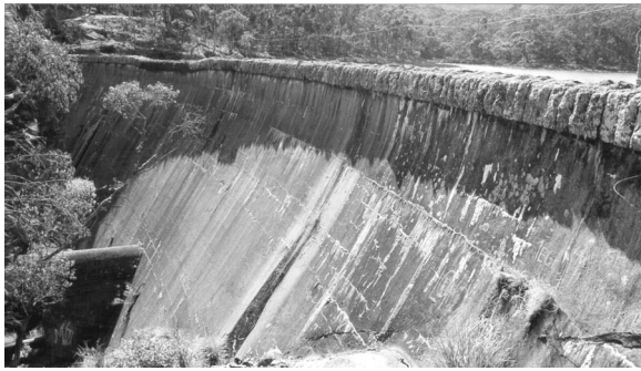
Fig. 2. January 30, 2000, photograph of the Lower Stony Creek Dam in Geelong, Australia (masonry dam completed in 1873): H = 18.3 m, L = 68 m. The dam was the first curved gravity dam in Australia. Note the low-flow spillway section in the middle of the dam crest.
