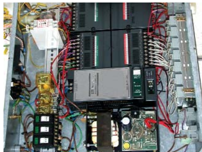
Figure 3. Programmable logic controller used to gather parameter data and regulate functions during autoclaving. The unit shown is from a prototype autoclave built by the author some two decades ago.
