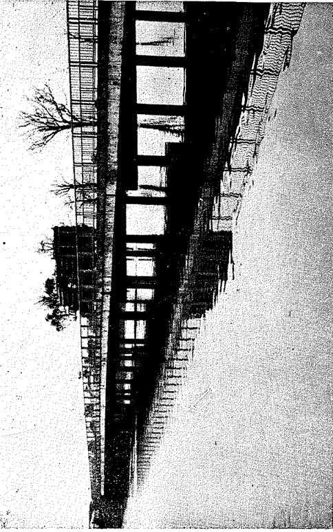
Slide 6. Nudgee Road Bridge 8th November, 1970. General view of bridge. No fixed debris.
