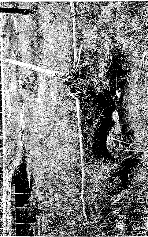
Slide 17. Scour round a telegraph pole near "Jerry's Downfall" culvert.
