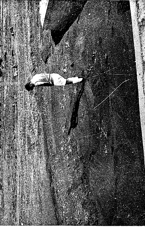
Slide 10. The upstream end of a single cell culvert showing the radiused concrete lip on which the C.D.W. engineer is standing.
