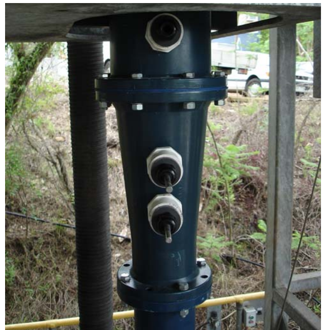
Figure 3, View of Krebs DF6 150 mm hydrocyclone used in velocity tests with tapping ports
