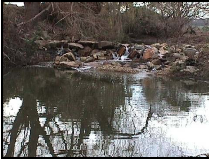
Figure 2 - Rock lost off the face of a rock chute on Iguana Creek, Mitchell River Catchment
