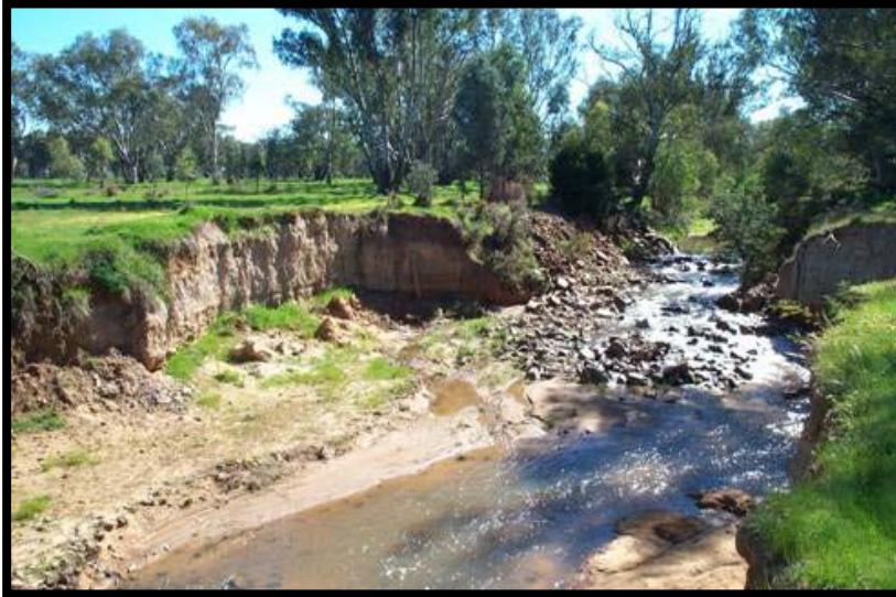
Figure 4 – The apron is being undermined on this chute but there is also downstream bank erosion and the danger of outflanking.
