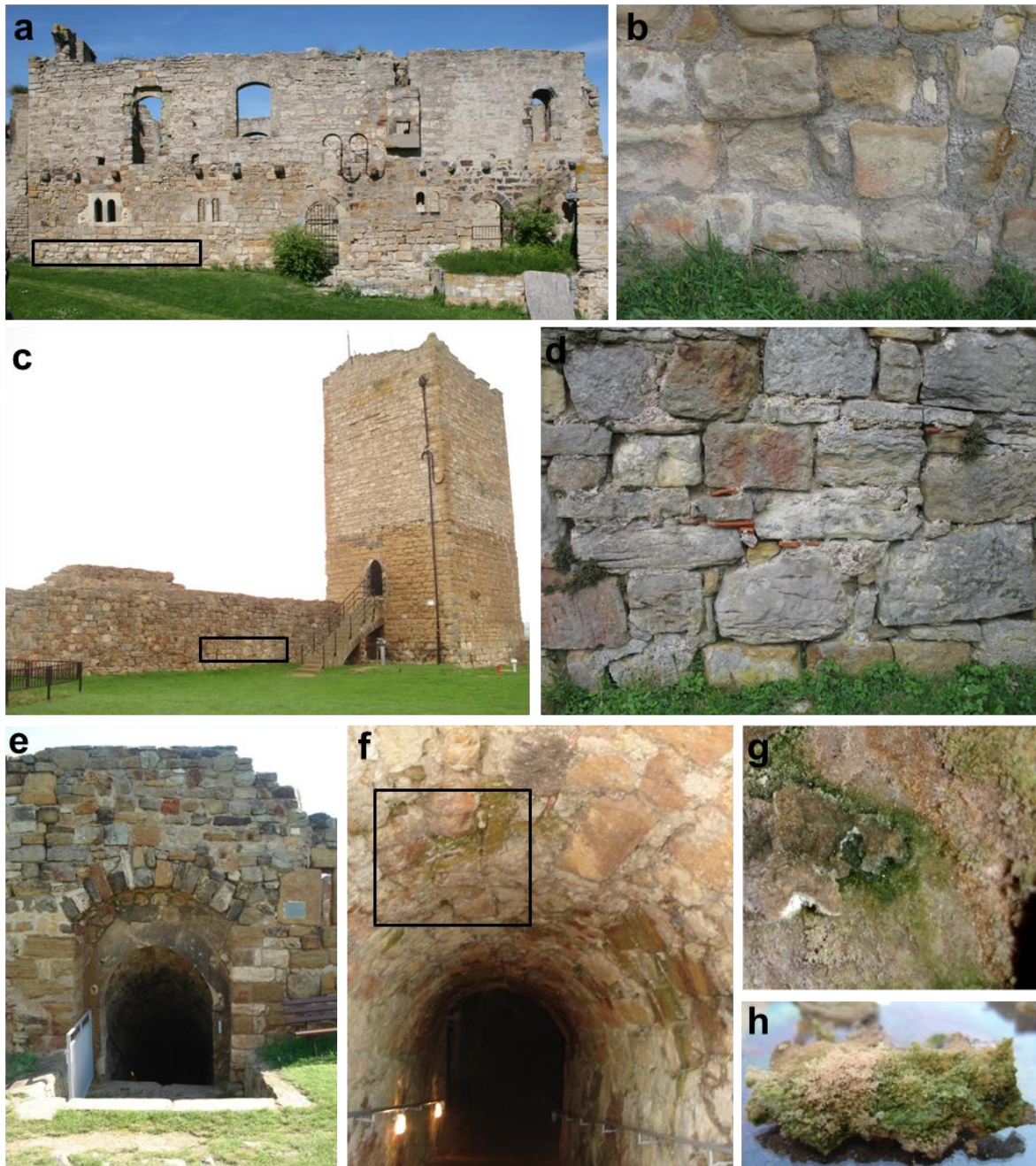
Fig. 1. Sampling sites on Gleichen castle. (a) Wall area A, sun-exposed. (b) Wall A in detail, with wall joints mostly filled with mortar. (c) Shaded wall area B. (d) Wall area B in detail, most wall joints open. (e) and (f) Dark basement vault, with scale samples removed from the basement vault. (g) and (h) Scales with green biofilm. Black frames: sampling areas.
