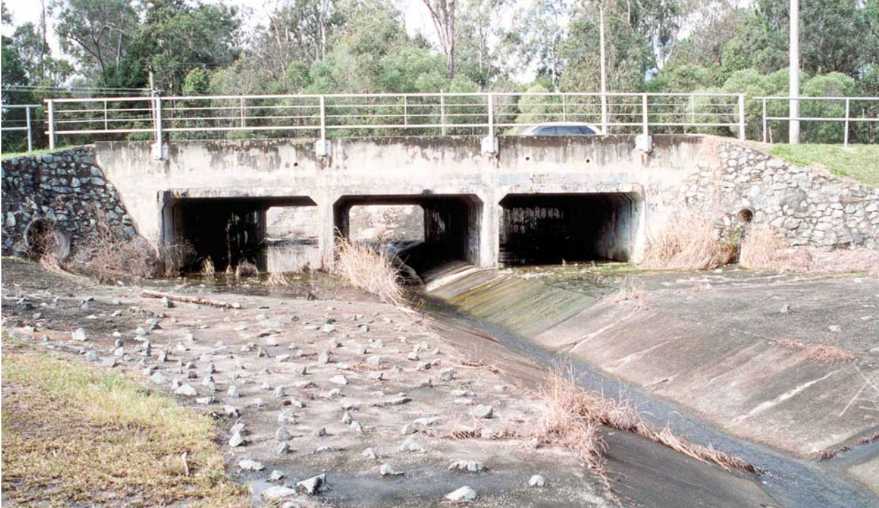
Fig. 1 - Standard culvert outlet at Algester Rd, Algester (Brisbane)
