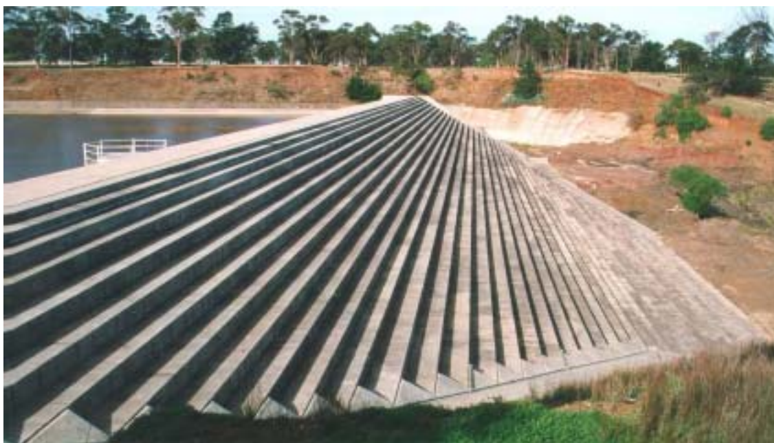
Figure 3 Melton dam stepped spillway on 30 January 2000—Completed in 1916, the Melton dam was equipped in 1994 with a secondary stepped spillway ( Q_{\text{des}} = 2,800 \text{ m}^3 \text{ s}^{-1} , h = 0.6 \text{ m} ).
