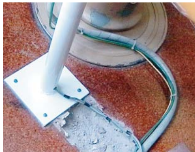
Figure 9. Surgery floors must be impermeable, a requirement not fulfilled in this case because of the cork tiles and the exposed uneven concrete. The electrical leads pose a trip hazard to staff as well as a potential electrical hazard.
