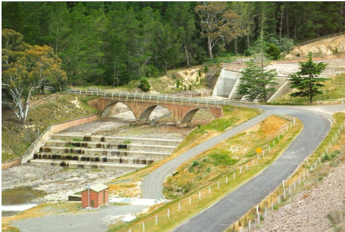
Fig. 1 - Upper Coliban stepped spillway (1903, Australia) 5 December 1997 (Courtesy of R. Smyth, Coliban Water) - Dam height : 30 m - View from the dam wall - Note the large drop upstream of the bridge and a series of smaller steps downstream
