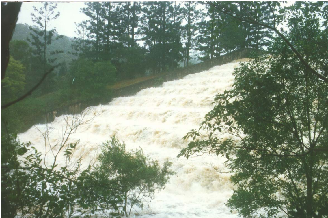
Fig. 4. Photographs of the Gold Creek dam spillway in operation (taken on 2 May 1996) (a) View from the left bank and downstream
