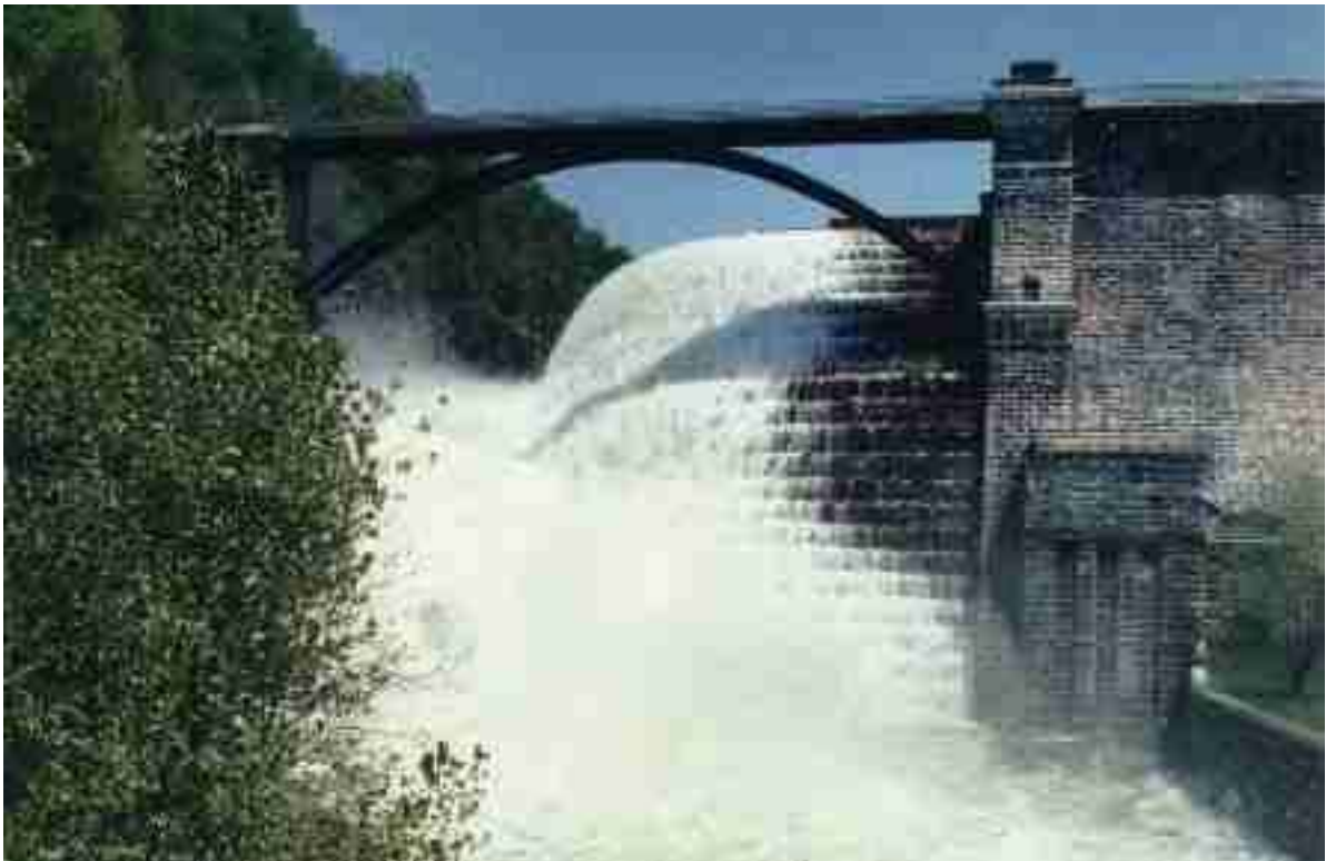
Fig. 3 - New Croton dam spillway (Courtesy of Matthew HILLER) - Recent photograph during a small overflow
