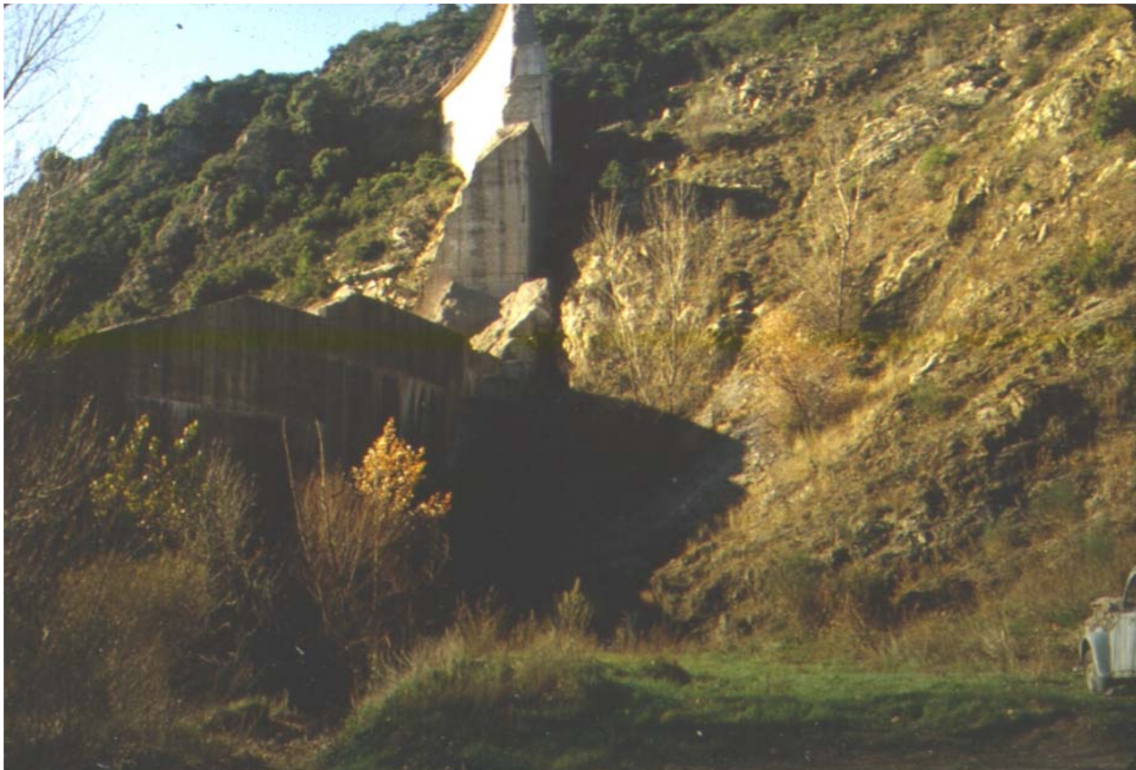
Photograph of the Malpasset dam taken in 1981 (Accident on 2 December 1959) - View from the reservoir looking downstream at the right abutment with the writer's car on the bottom right for scale
