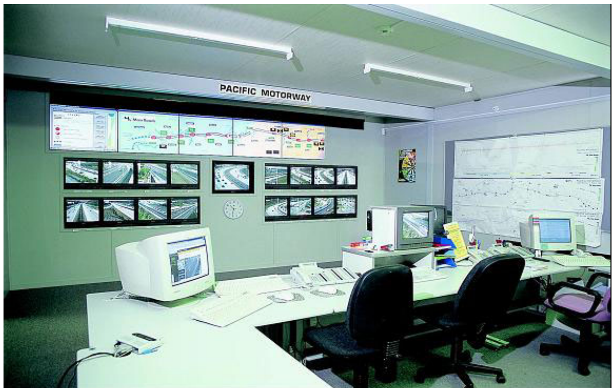
Figure 3 – Project Traffic Management Center
