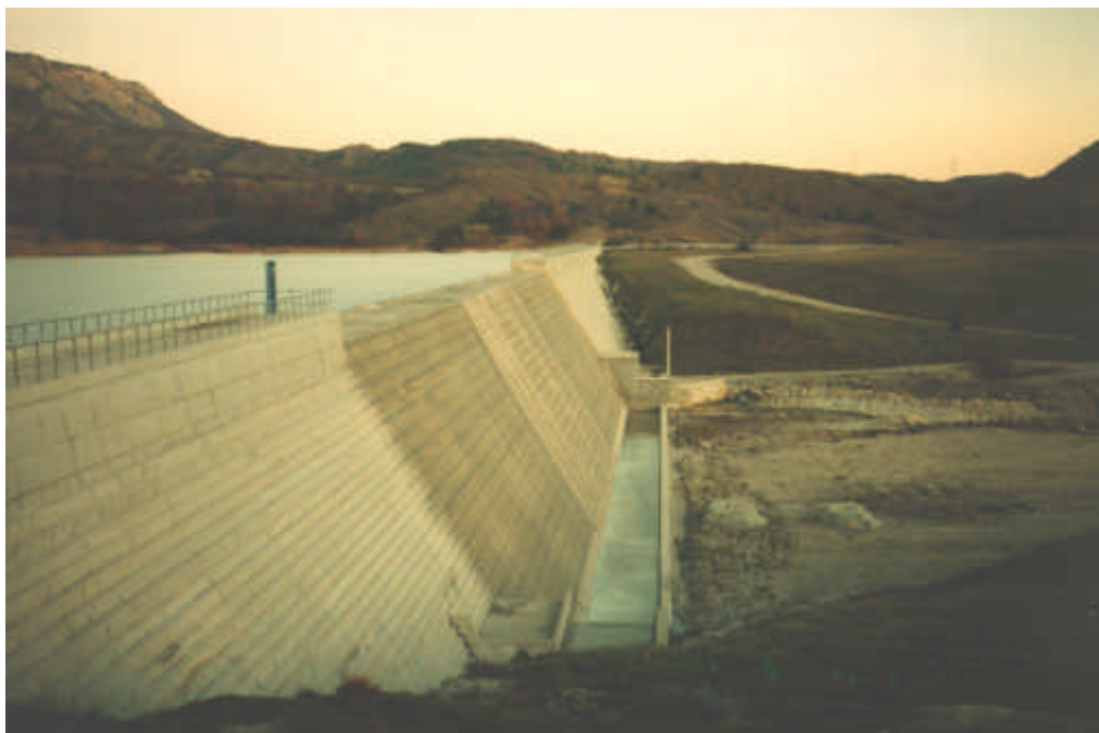
Fig. 1-1 - Photographs of stepped spillways (B) Riou dam, France in November 1994 - Completed in 1990 ( H = 22 m), design discharge : 1.5 \text{ m}^2/\text{s} , width : 96 m, h = 0.43 m, RCC construction
