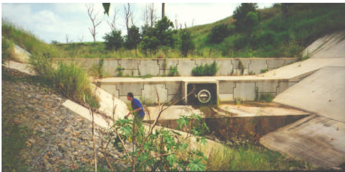
Fig. 7-3 - Earthfill embankment with a rockfill upstream protection and reinforced earth downstream slope construction : Jordan II, Gatton QLD (Australia, 1992) on 22 Feb. 1998 - H = 5.3 m, h = 1.4 m, \alpha = 17.7^\circ - View from downstream
