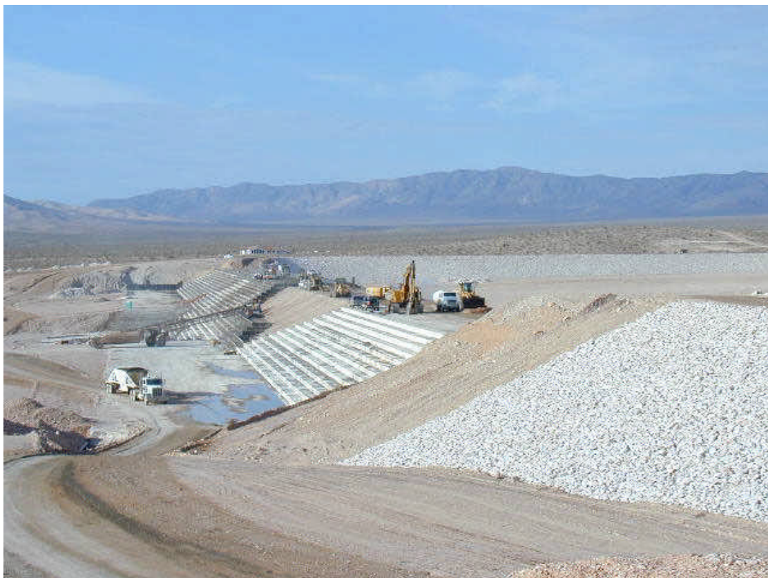
(B) Construction of a RCC spillway for detention basin West of Las Vegas, designed by the US Corps of Engineers
