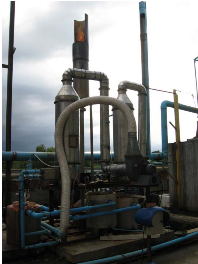
Figure 2.2 The Pilot packed column used in H 2 S removal from biogas process
