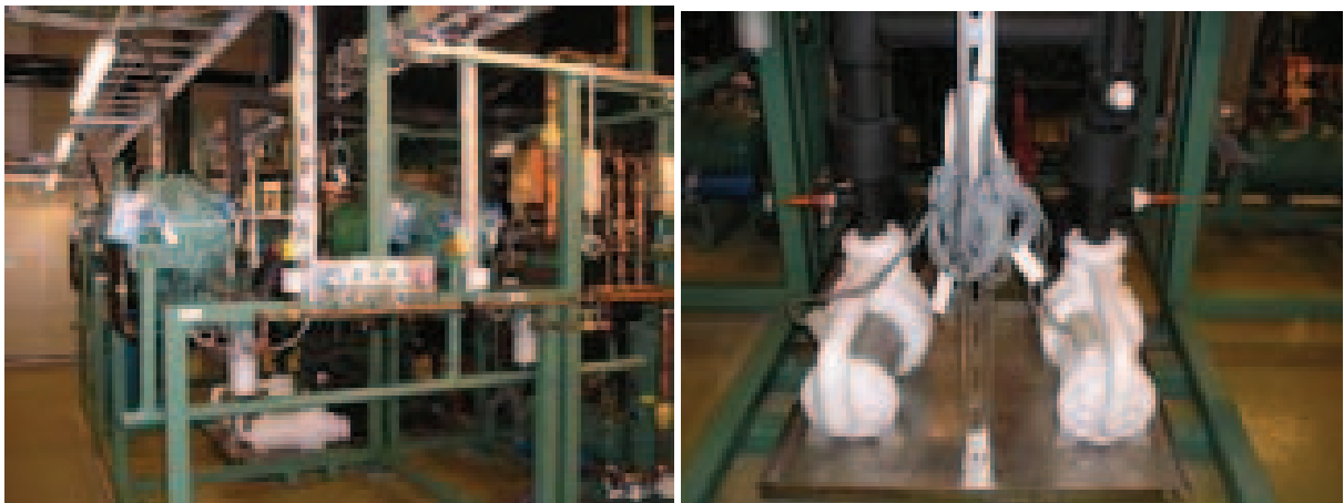
Fig. 4. Machinery room views.
