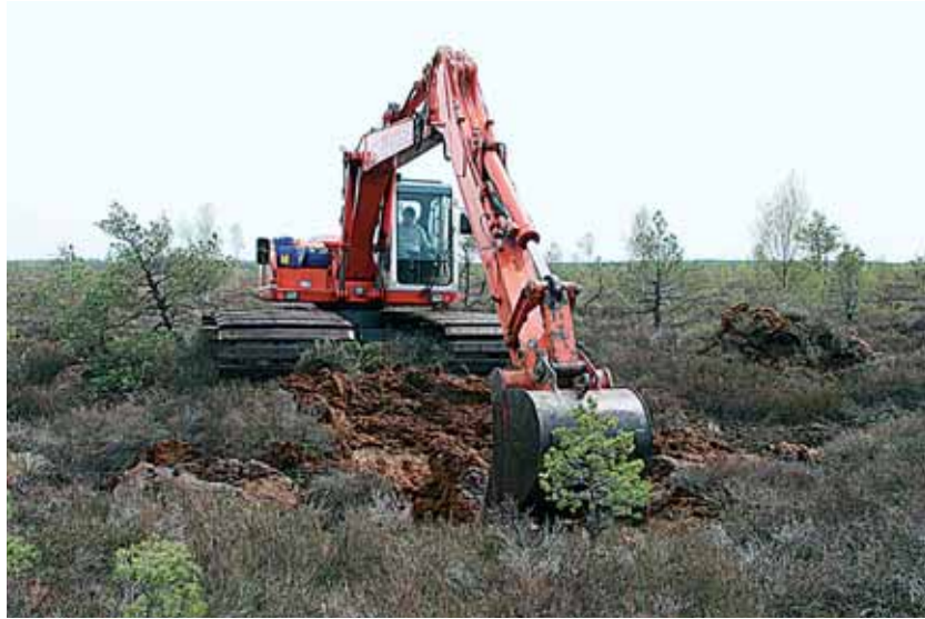
Figure 6. Building of dams in drainage ditches in Cena Mire (Photo M. Pakalne).
