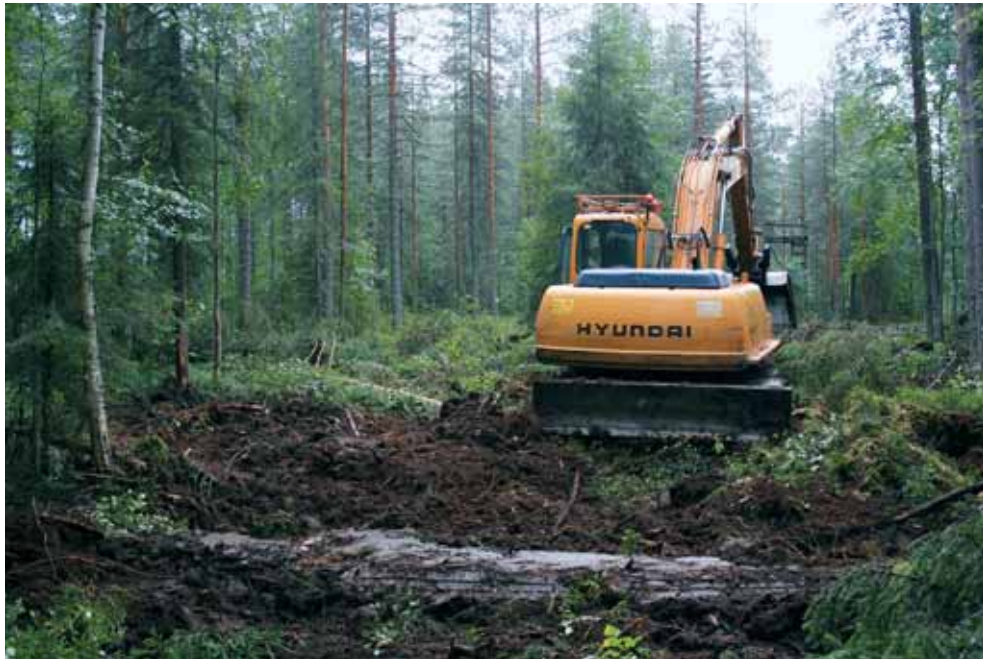
Figure 1. After several unsuccessful attempts to restore drained peatlands by damming the ditches with hand-made dams, it was realized, that the only way to do it efficiently in large scale would be to use machinery. Excavators can be used to fill-in the ditches tightly in both semi-open and forested sites. Photo Maarit Similä, 2.8.2006, Koitajoki Natura area, East-Finland.
