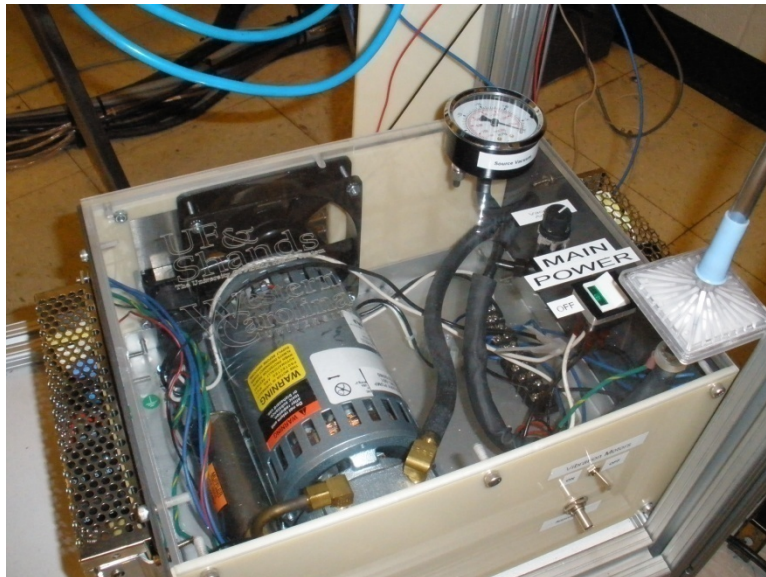
Photo of electrical component box.
