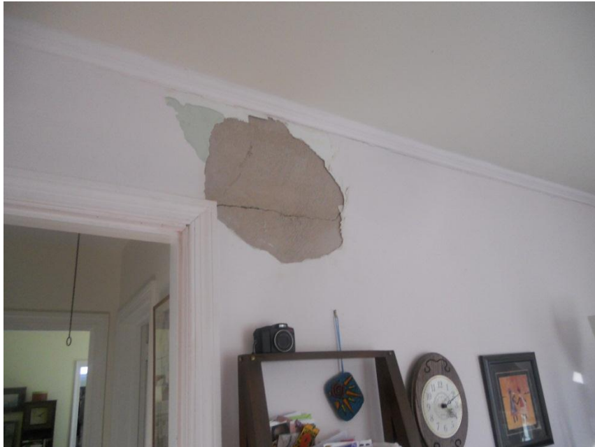
Figure 21. House #2 Bedroom. Several large cracks can be seen in the original plaster of the second bedroom (Source: Author).
