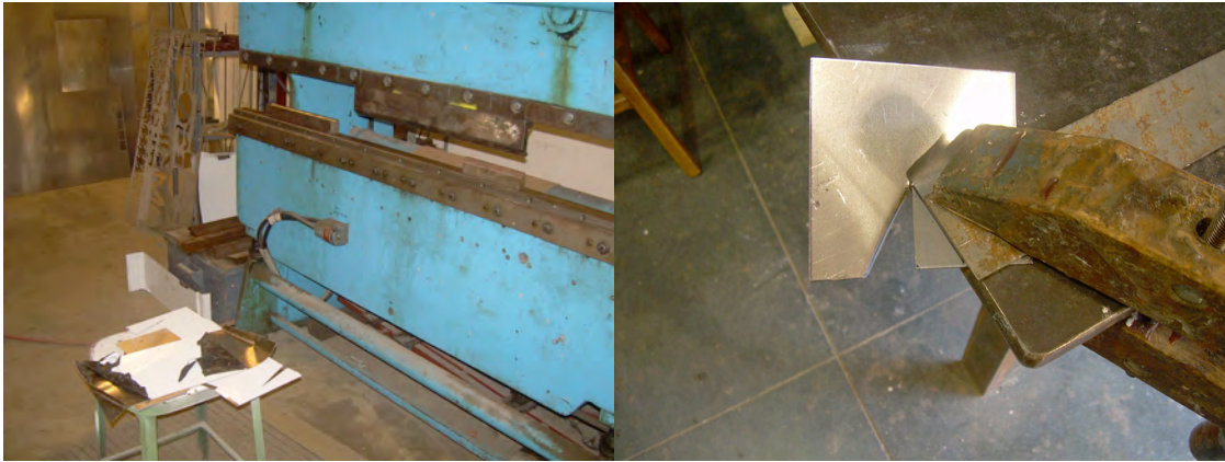
Figure 65: Left side: breaking the sheet metal with an industrial brake. Right side: cold bending by hand.
