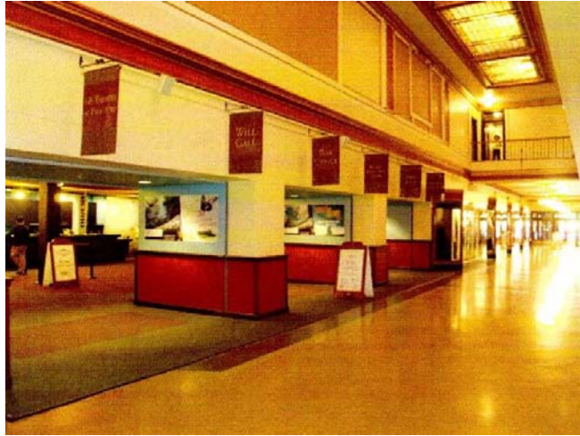
Figure 11. Proctor's Theatre, arcade west wall was removed to gain access to the adjoining space (now part of theater interior); affected form, proportion, rhythm, and scale
