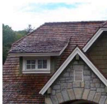
The materials used in the roofing here are multi-colored with different shades of brown and gray. The color and texture are visually appealing and in harmony with the surrounding natural environment.
