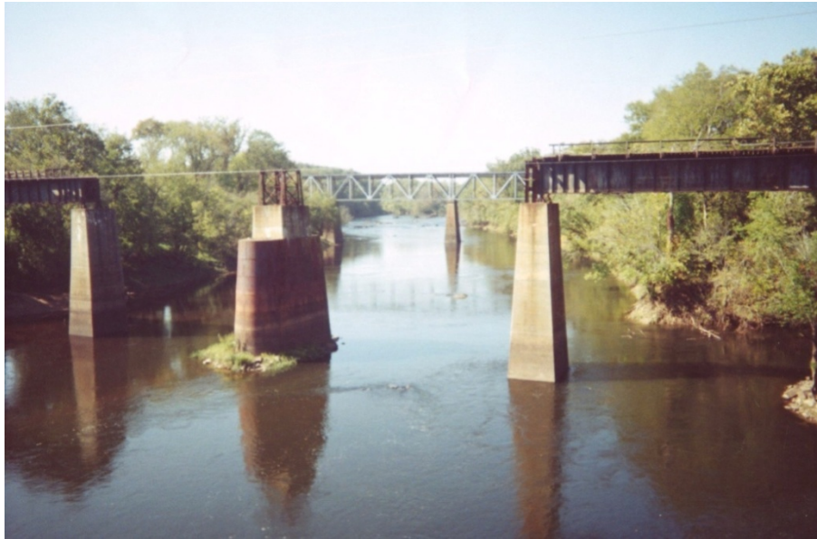
Figure 22. The abandoned Seaboard Coastline Bridge over the Roanoke River at Weldon is located at the site of the Weldon Toll Bridge. Photograph by Cynthia Johnson in November 2000. Copyright owned by James C. Burke.
