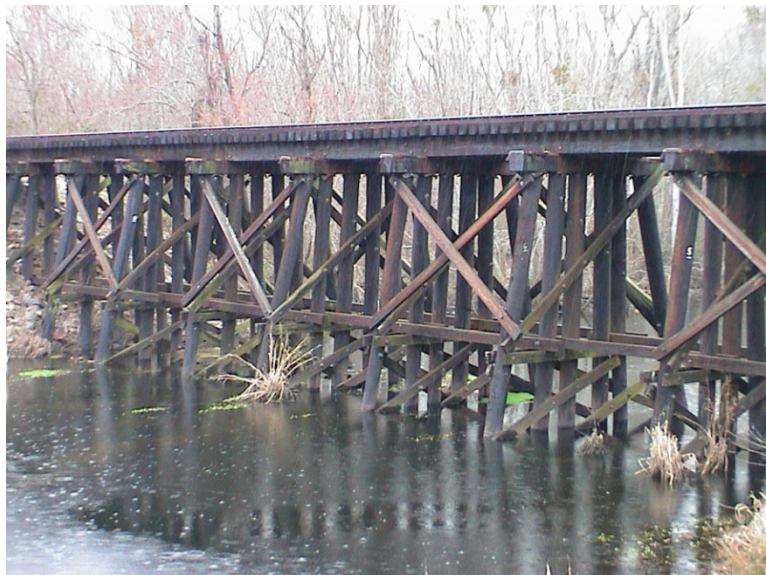
Figure 8. Modern trestlework is used on the railroad at Goshen Swamp. The method is still practiced in railroad construction, and this example resembles the description of the high trestles on the Charleston & Hamburg Rail Road in many aspects. Photograph by James C. Burke
