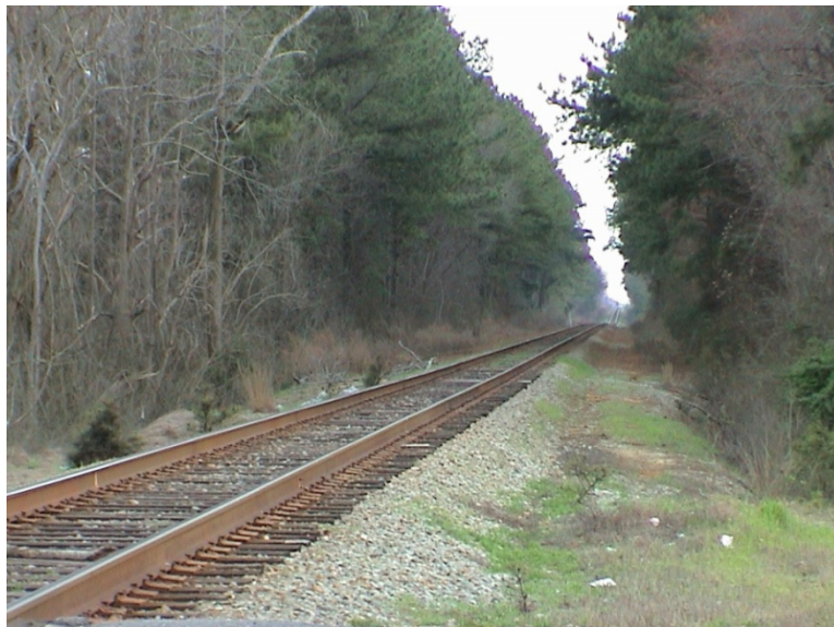
Figure 10. This photograph, taken at Brogden looking south toward Dudley, shows how the track follows the undulations of the terrain. There are several deep cuts in this section. Photograph by James C. Burke
