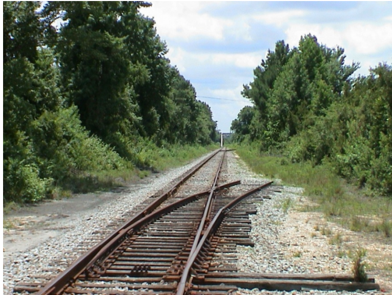
Figure 3. This photograph, taken on the north side of Smith Creek in New Hanover County, NC, illustrates the level character of the alluvial land of the Lower Cape Fear. The modern railroad track is set in a modest layer of ballast. Photograph by James C. Burke
