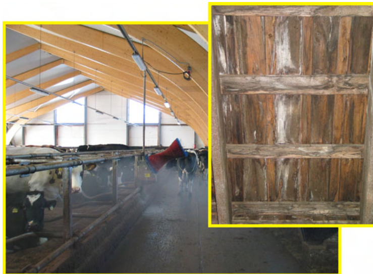
Figure 13. Moisture and mold observed in some of the dairy buildings measured.
