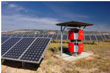
Figure 3: System 2 facility situated at Herrera de Valdecañas (Palencia, Spain)
