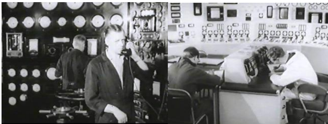
Figure 2-4. Power station control room before and after the implementation of ergonomic design principles. 165
