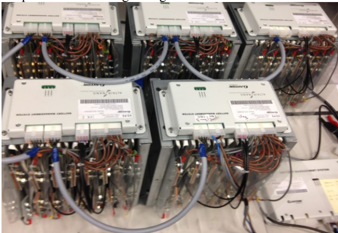
Fig. 5: Implementation of the battery stack consisting of 5 modules with 15 Altairnano 13Ah cells each.
