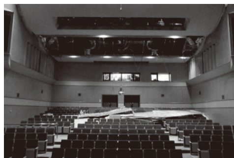
Fig. 2 Ceiling collapse occurred during 2016 Kumamoto Earthquake 2)
