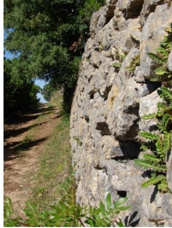
Fig. 3. Supporting wall in Algarvian barrocal , where one can observe the slope in the parament, to compensate the pressure of the terrain (Source: authors)
