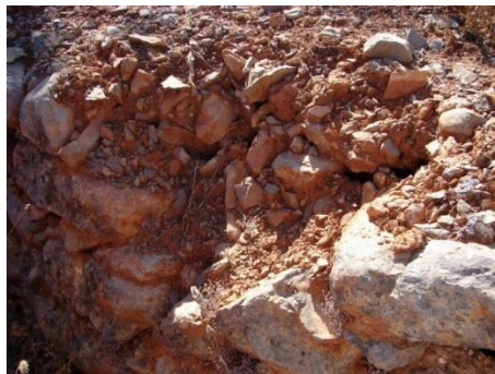
Fig. 4. Wall in the Algarvian barrocal , partially destroyed, where one can see the filler of the wall with stones of smaller granulometry (Source: authors)
