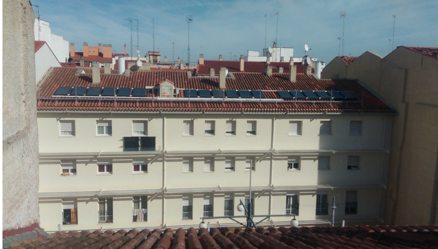
Fig. 7 Building A after intervention facade insulation, incorporation of sunscreen, hybrid solar panels for hot water and electricity, solar lighting conduits for patios and prototype passive solar heating.
