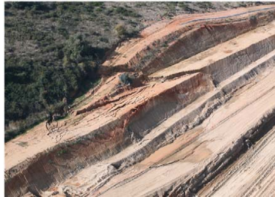
Figure 2.- Observed failure during construction
