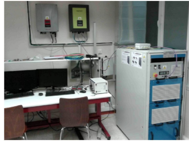
Figure 6: Li-ion Battery demonstrator
