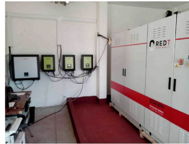
Figure 5: Vanadium Redox Battery demonstrator
