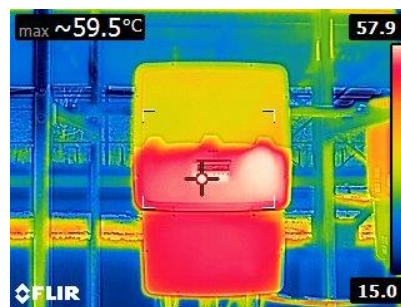
Figure 8: Inverter operation conditions
