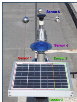
Figure 2: Environmental sensors mast.
