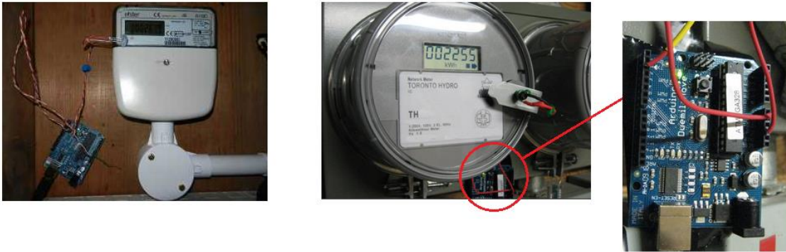
Figure 3. Smart meters using proprietary devices combined with Arduino Uno [11] boards
