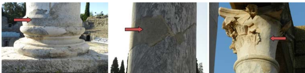
Fig. 3. Restoration mortars used in different periods for the structural consolidation of the Front stage in the Roman Theater of Merida (Photos by Natalia Perez)
