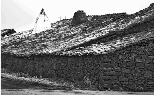
Figure 1. The forms of the architecture are adapted to the natural and human media. Dwellings in Villaciervitos (Soria, Spain) are grouped in rows. They have a big roof with low slope. Northern walls are low and thick and they have not hollows. In the interior there are coexistence of humans and animals. The big chimney (called chimenea pinariega ) covers the whole of the space of the cook room (Gil Crespo).
