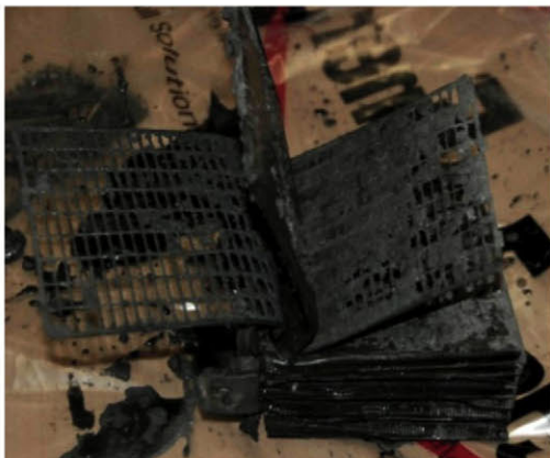
Fig. 10. Loss of active mass in the positive plates in one of the cells of the battery.
