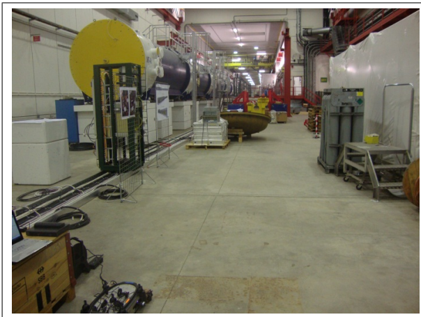
Figure 2. ECN3 tunnel area at CERN - location of the transmitter (Point A in figure 6)
