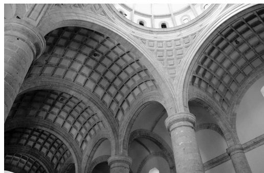
Fig.3: Vaults of Cathedral of San Ildefonso, Yucatán, México. Ribs with distorted section.
