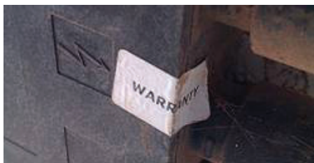
Figure 5: Sealing label of “warranty” in the junction box of a PV module.
